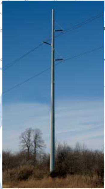
The structure shown here will be used for the majority of the new transmission line. Some portions may include the placement of local distribution lines on the same poles.
