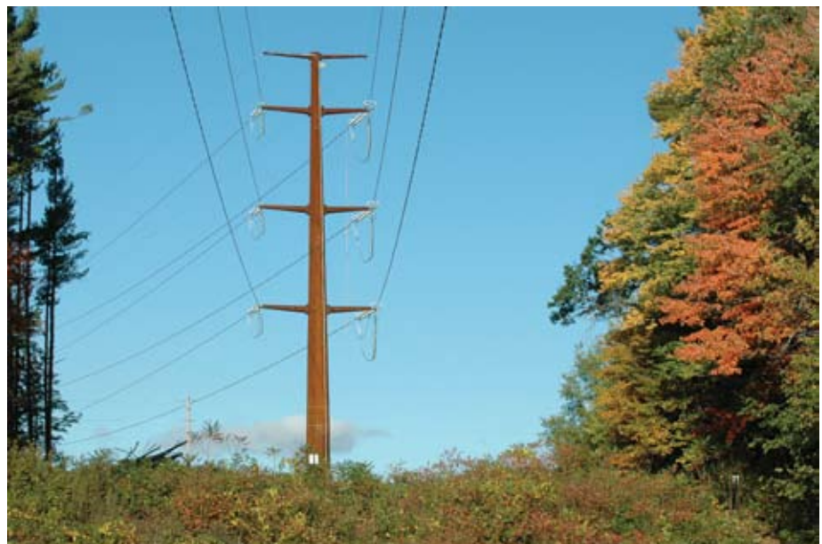
A view of the transmission line west of Shawano. This portion of the project was completed last fall. See the map inside for details on all project segments.
