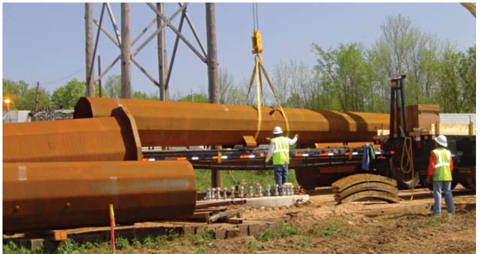
A crane prepares to lift part of a transmission pole off of a flatbed to install along the right-of-way.
