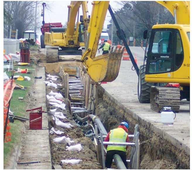
Taken from another project where ATC buried transmission lines underground, this photo illustrates the type of work that will take place on the Cranberry-Conover segment of this project.
