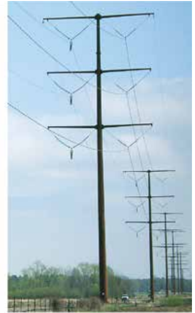
Double-circuit weathering steel A typical design of a double-circuit weathering steel 345-kilovolt transmission line that may be used for the project.
