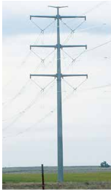
Double-circuit galvanized steel A typical design of a double-circuit galvanized steel 345-kilovolt transmission line that may be used for the project.
