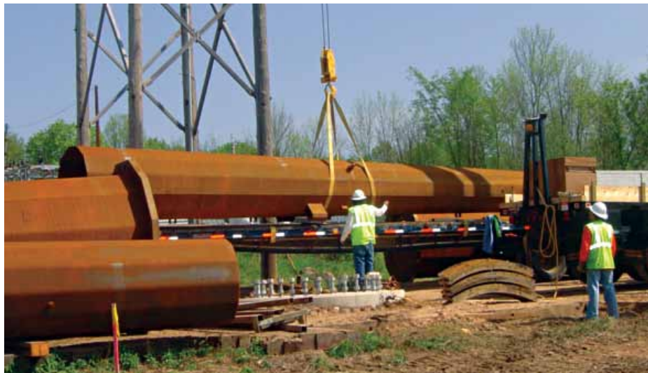
A construction crew uses a crane to lift part of a transmission pole for installation along the right-of-way.
