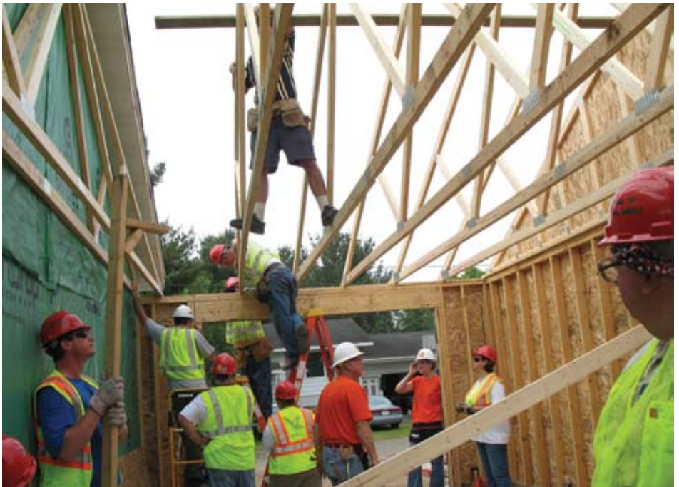
Volunteers set the last truss, which is a triangular unit that connects at the end with joints. It was an integral part of the garage that was built.
