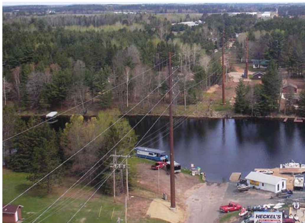
Some of the tallest poles on the project – 115 feet – were used to cross the Eagle River.
